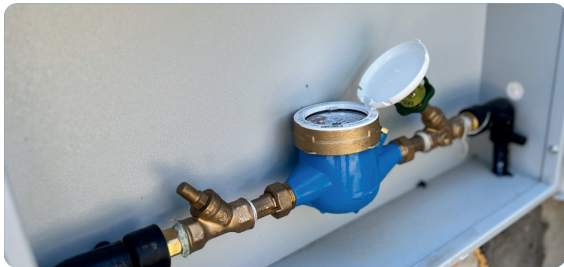
Individual water meters for households are key for fair, transparent and just invoicing of water consumption.
