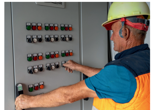
Control board of the rehabilitated water reservoir Krasta e Madhe.
