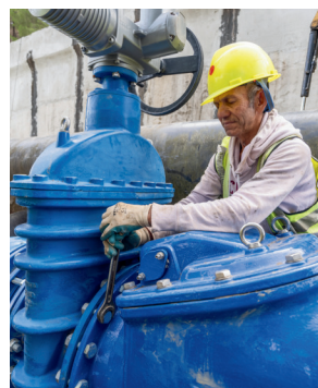
Installation works of a new pump for the rehabilitated water reservoir Krasta e Madhe
