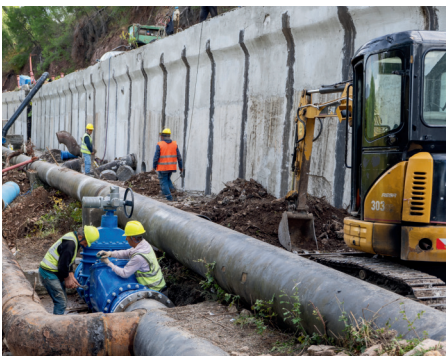
Construction of the new water reservoir Krasta e Madhe, which will contain 2,000 m 3 of fresh and clean drinking water
