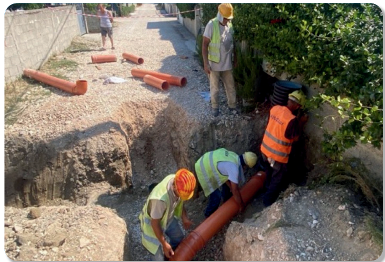
About 700 households have been newly connected to the public sewerage system of Fier
