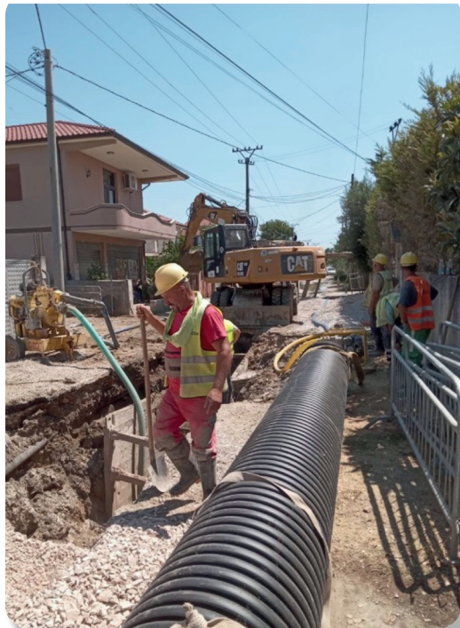
Huge main collector pipes for waste water collection
