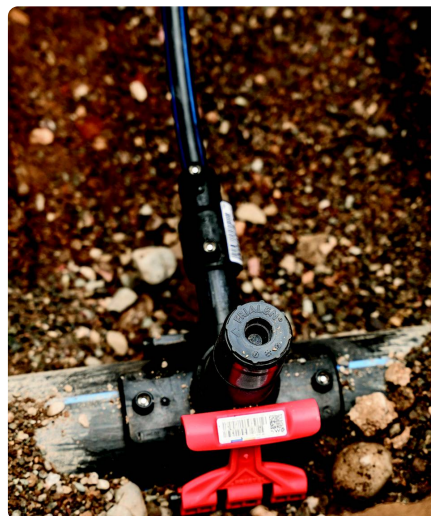
Individual household water supply pipe (small diameter) connected to a wide diameter distribution pipe.
