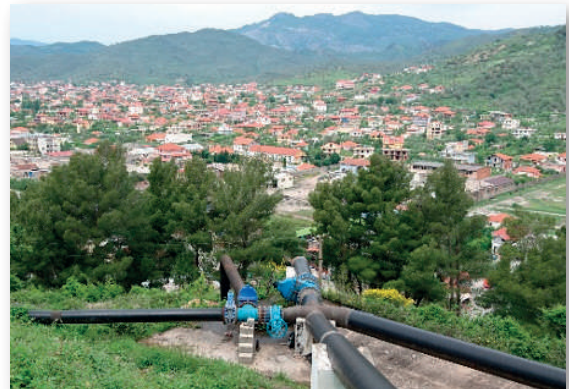
Water pipe from reservoir Krasta e Madhe
